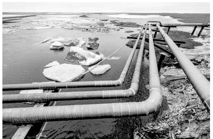
Pipelines extend across the landscape outside Nuiqsut, Alaska, May 2019.
